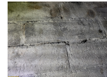
firebox cracks .jpg firebox cracks .jpg
