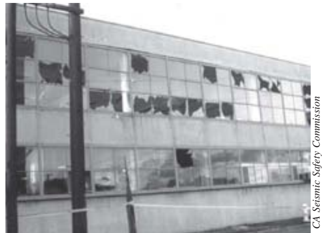
Figure 56 —The windows in this San Francisco building probably broke because its frame flexed too much in the Loma Prieta earthquake of 1989.
