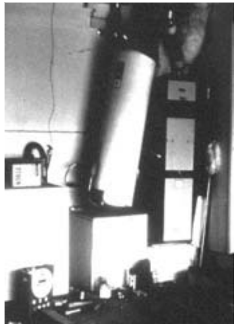
Figure 11 - This unstrapped water heater tipped over during the 1984 Morgan Hill Earthquake. Fortunately gas and water lines were not ruptured.
