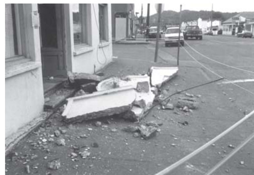
Figure 20 - Unbraced Parapets can Injure and Kill - This parapet on the front of the building in Figure 18 fell on the sidewalk.
