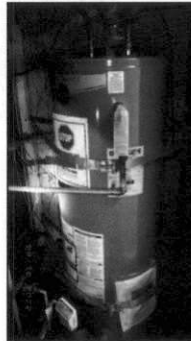
newer water heater
