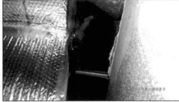
missing fire wall
