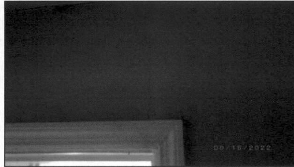
typical settlement cracks
