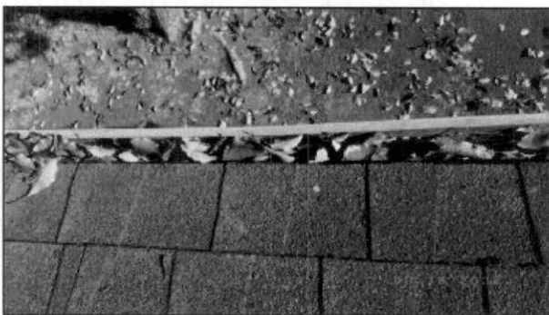
debris in gutters
