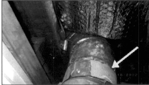
possible asbestos material
