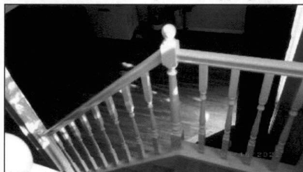
openings too big
