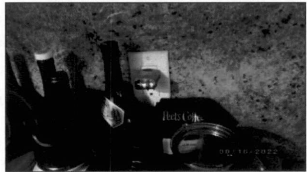
missing GFCI protection
