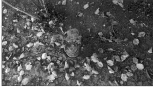
sewer clean out
