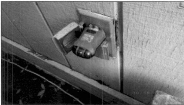
missing GFCI protection
