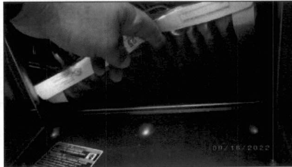
dirty and wrong size
