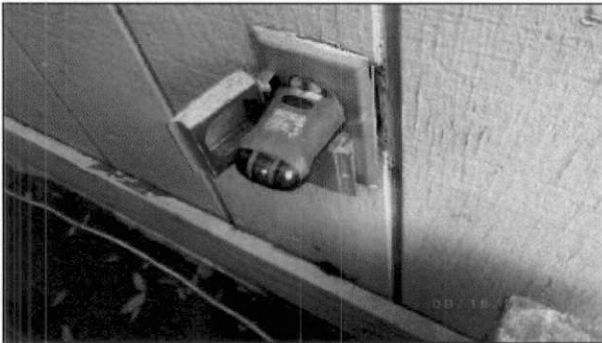
missing GFCI protection
