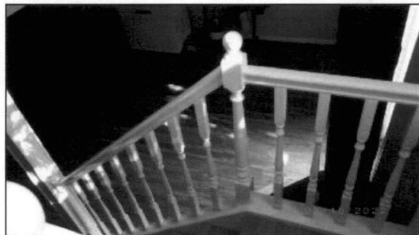
openings too big
