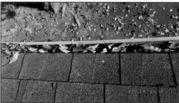
debris in gutters
