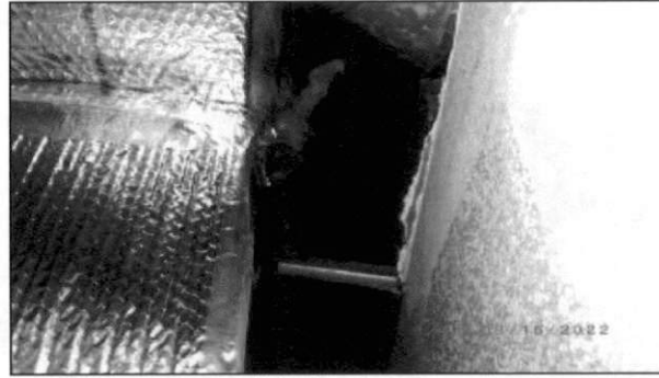
missing fire wall
