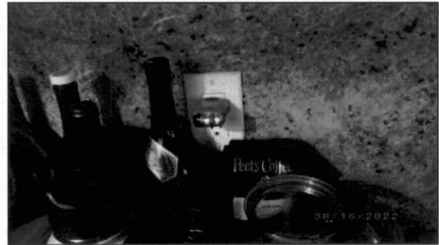
missing GFCI protection
