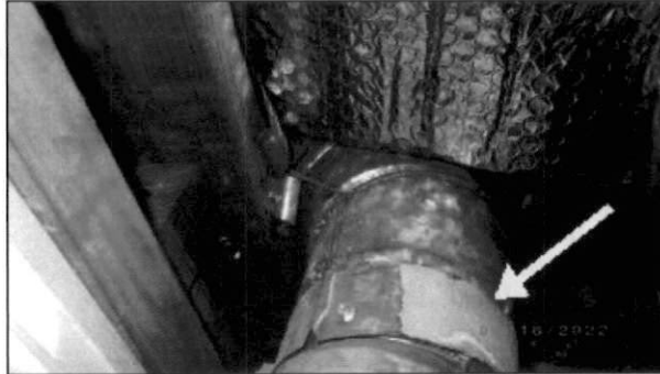
possible asbestos material
