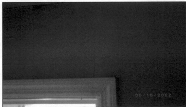
typical settlement cracks
