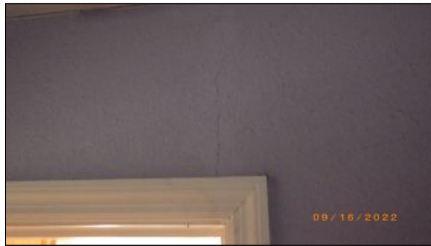
typical settlement cracks
