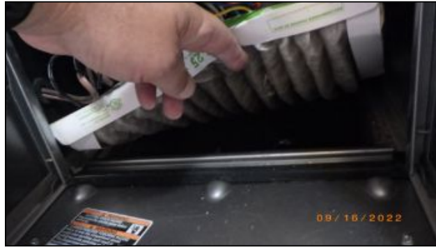
dirty and wrong size
