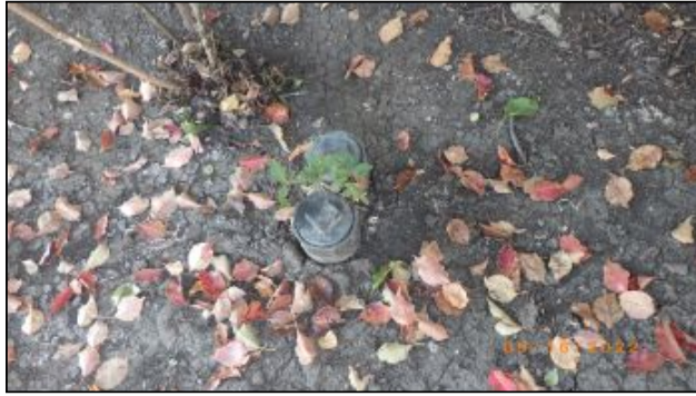
sewer clean out
