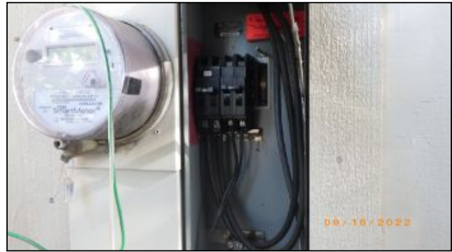
missing inner cover
