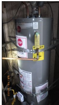
newer water heater
