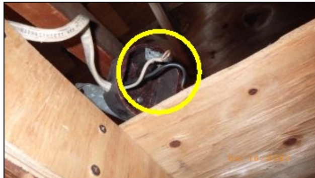
live uncapped wires
