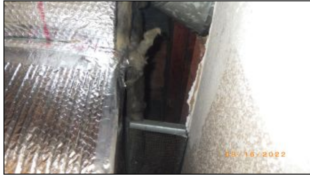
missing fire wall
