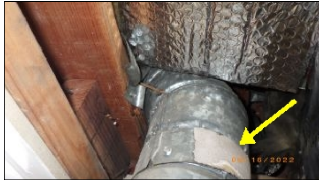
possible asbestos material
