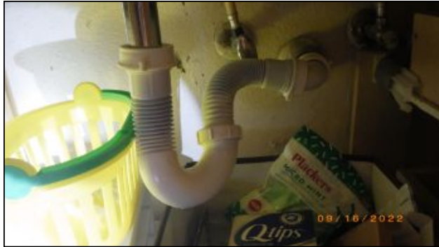
flex pipe used
