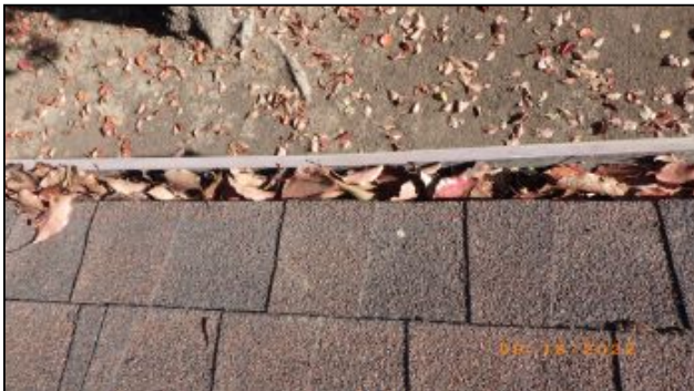
debris in gutters
