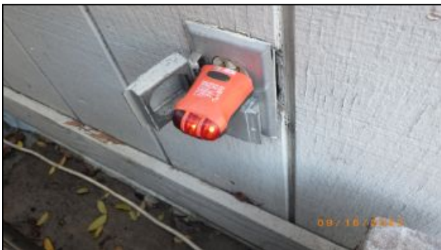
missing GFCI protection
